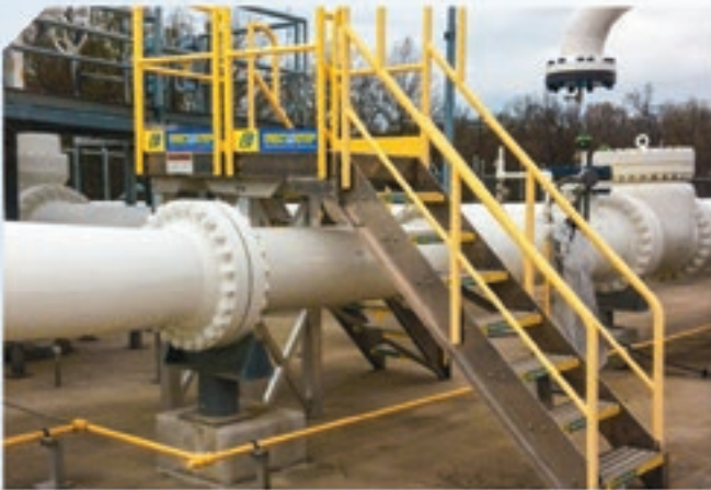
Large oil pipeline cross over.
