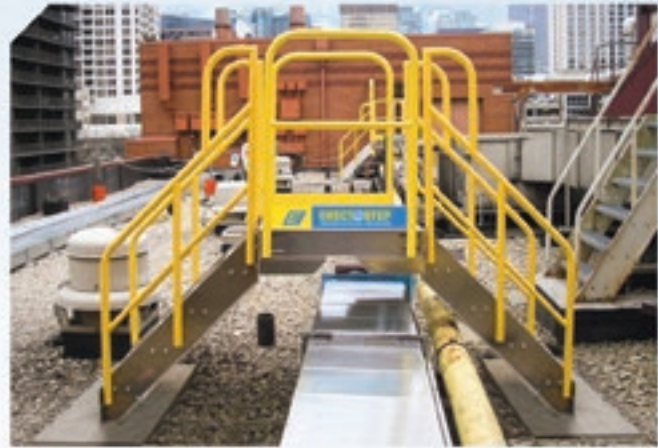
Crossing rooftop HVAC ductwork safely without damage to the lines.
