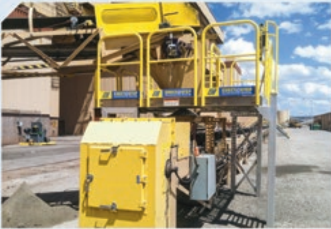
Work safely on all four sides of this conveyor motor at this power generation station.
